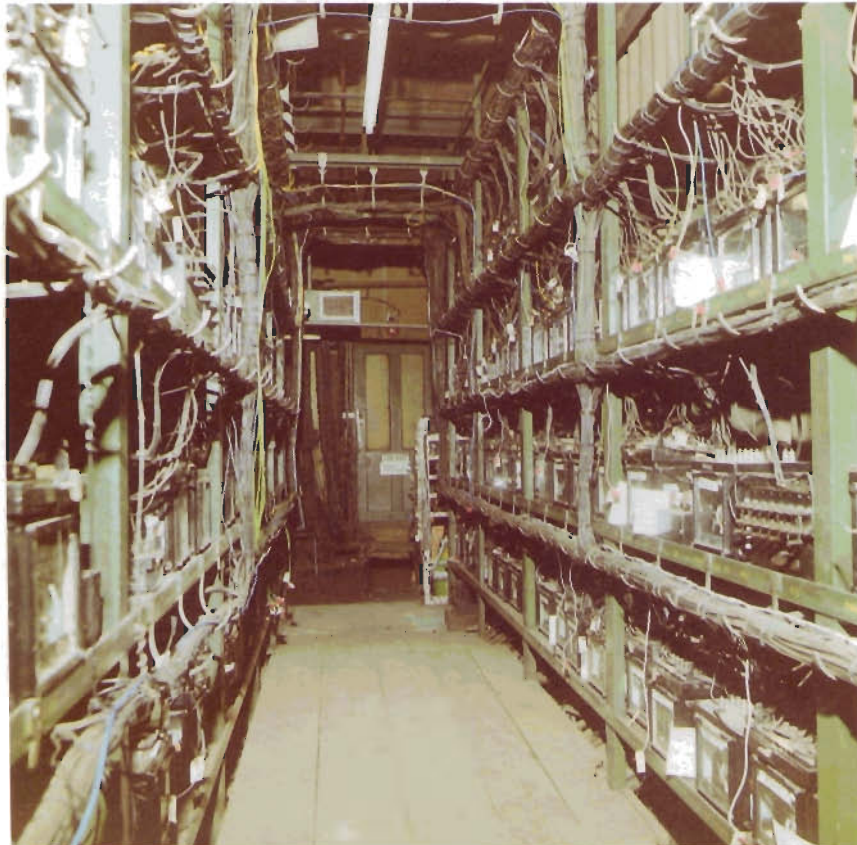
Fig 11. A view of the relay room, looking towards the entrance, showing the relay racks, and the trees of the wiring. Relays TRR DM and TRR DN are on the bottom shelf on the right in the last section towards the door.
